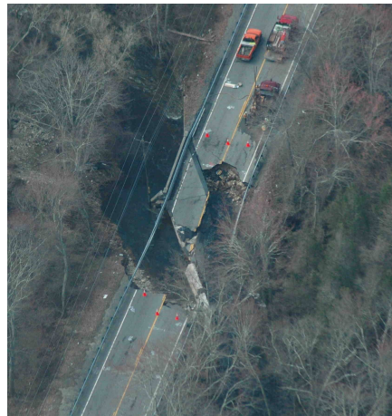
Rte 184 Bridge Failure near Old Mystic
